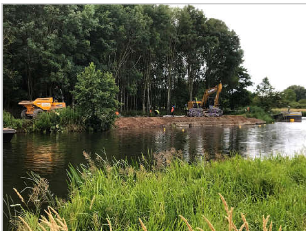
Now completed, but work in progress stabilising the river bank where the high-pressure gas main crosses the river.
