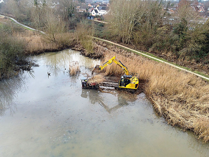
↑ Digger clearing reeds on 14 Jan 25 using a special bucket for this work. Picture courtesy of Wychavon DC
