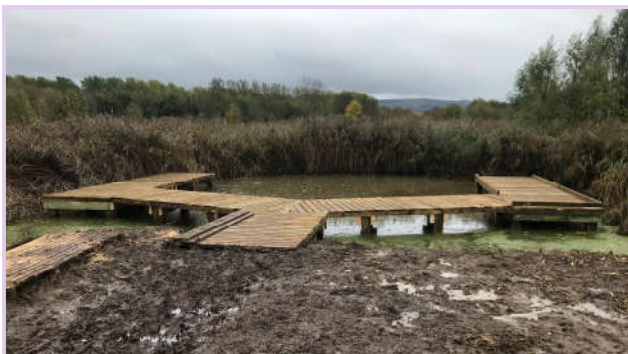
The new pond dipping platform under construction on 27 October. Designed by Wychavon engineering department.
